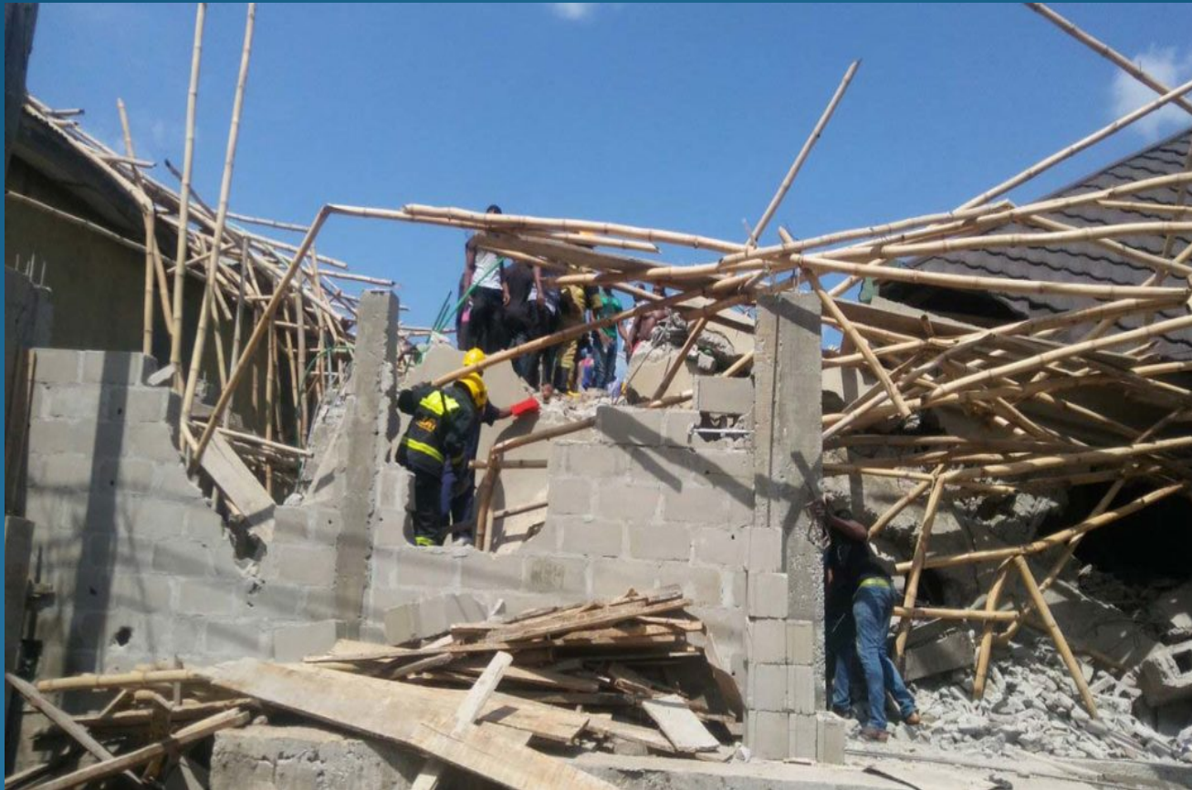
Collapsed Building in Lagos. Photo: Tobi Awodipe. Source; The Guardian
