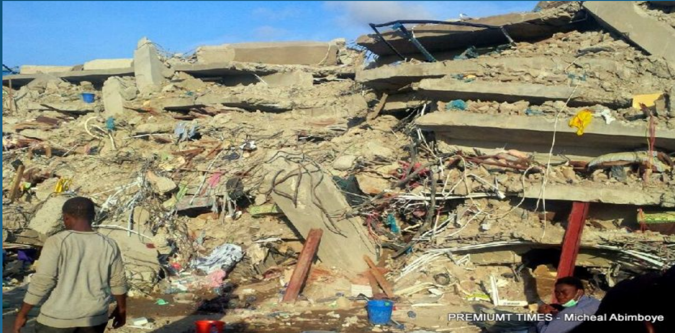
Collapsed Guest house at Synagogue church premises, Lagos.
